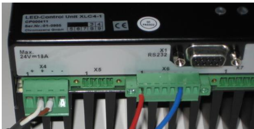
Figure 11: Detail view of the XLC4 controller showing the X6 port with cabling for single signal flash mode
